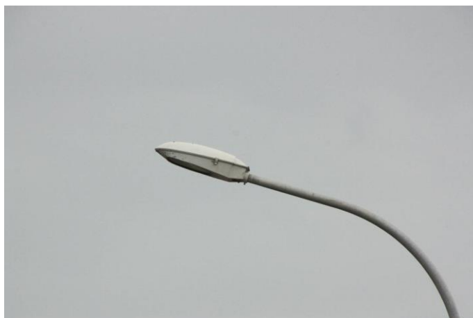
Armature installate in maniera errata
